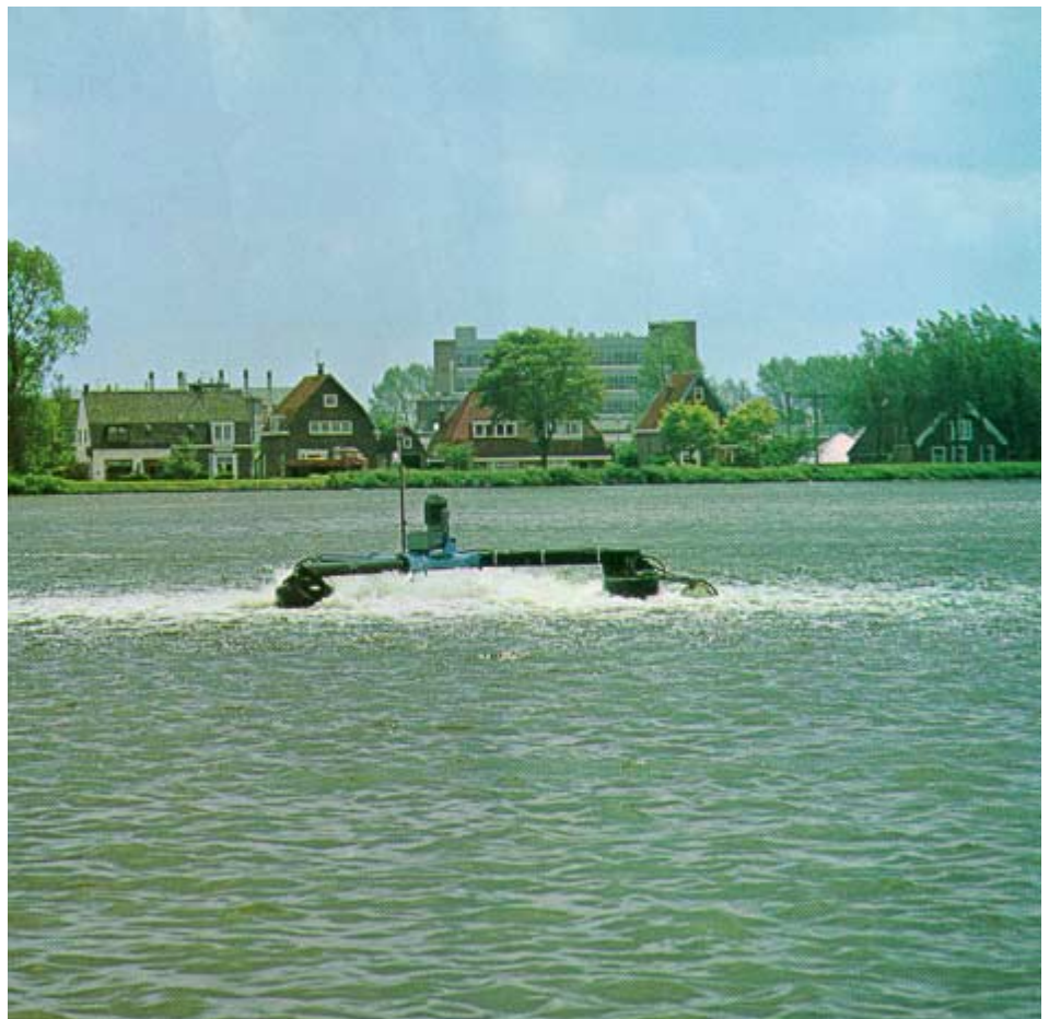
Fig. 26.10 Three-phase geared motor of vertical mounting on an agitator in a harbor filtration plant.
