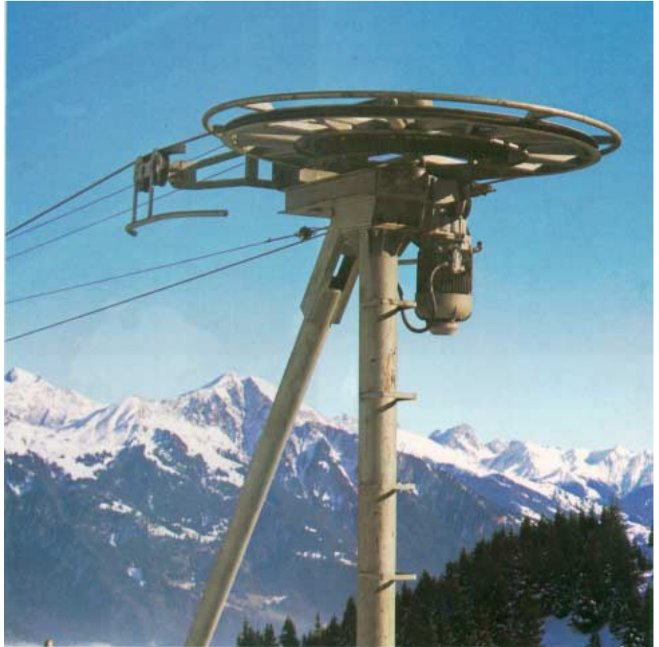
Fig. 23.2.3 »Outdoor installation« cannot be avoided for a skilift drive. The long idle periods are as critical as the effects of snow, ice and rain
