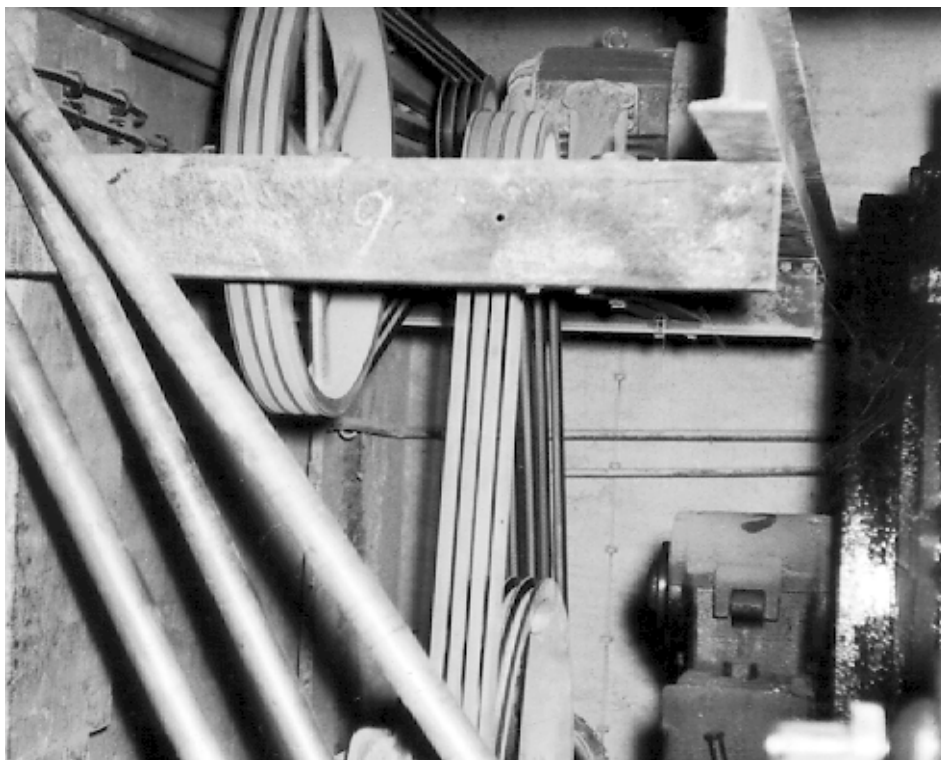
Fig. 1.2 Indirect drive of a wet drum grinder in a ceramics factory with standard motor and two-stage V-belt reduction
