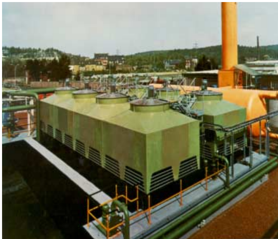
Fig. 19.4.1 Three-phase geared motors with special degree of IP66 protection (with extra protection against corrosion / CORO 3), driving a group of cooling tower fans
