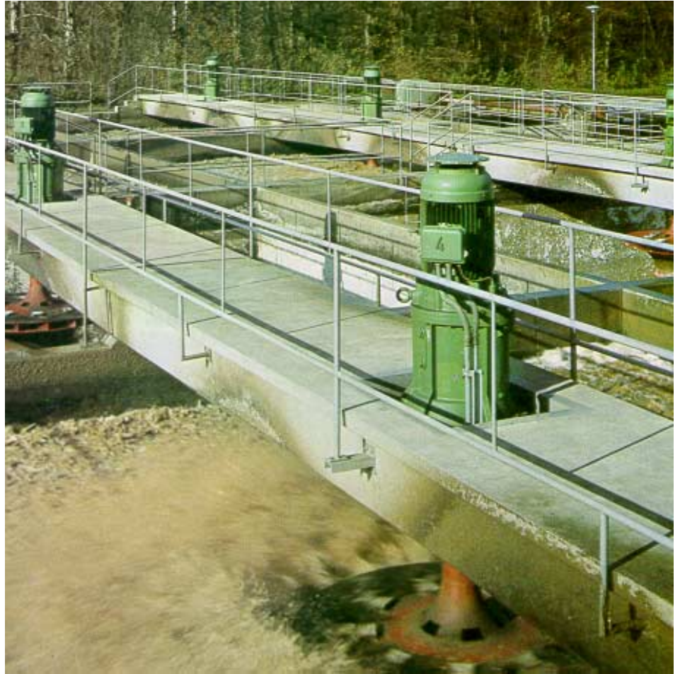
Fig. 26.28 V 1 arrangement of geared motors, driving aerators in a sewage treatment plant.
