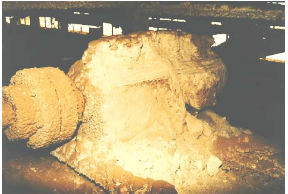
Fig. 15.2.2 Geared motor under “dust blanket conditions” in a malt factory
