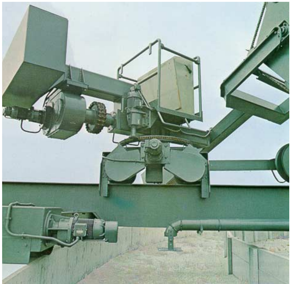
Fig. 26.8 Three-phase geared motors of various types in a sewage tank scraper.
