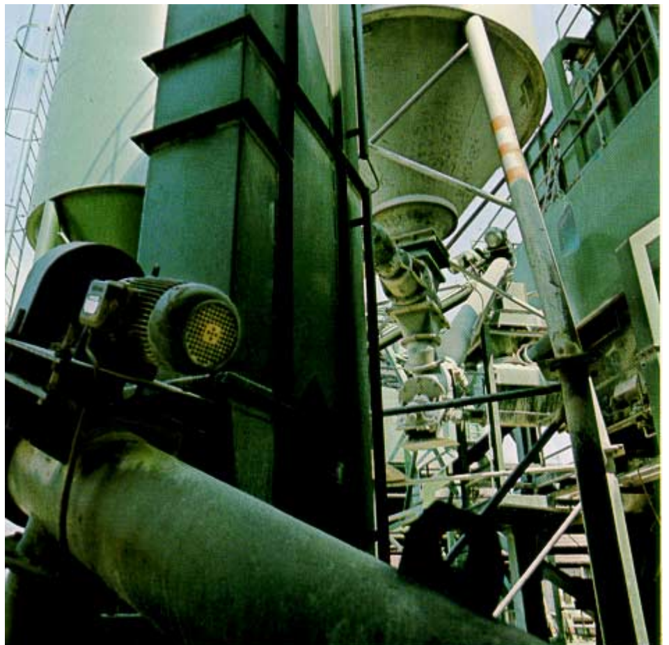
Fig. 26.12 Three-phase motors in a tar- macadam mixing plant.
