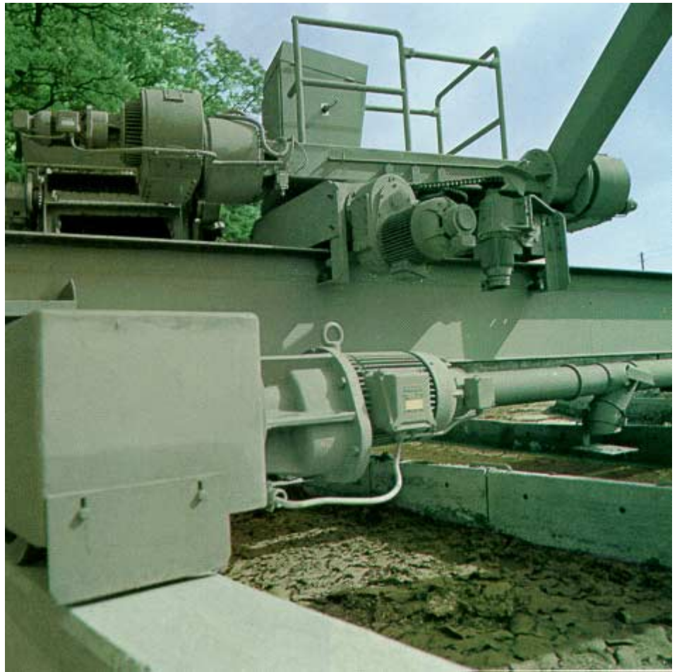
Fig. 26.9 Three-phase geared motors of various types in a sewage treatment plant.
