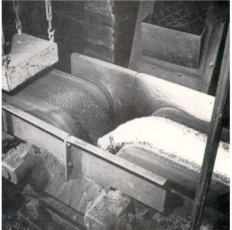
Fig. 26.20 Three-phase drum motors driving conveyors for the mixing of ores and salt in a copper plant.
