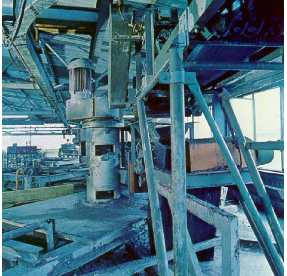
Fig. 26.13 Three-phase of geared motors various mounting on an acid mixing plant.
