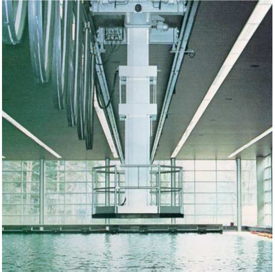
Fig. 26.24 D.C. geared motor driving a variable-speed swimming pool training gantry.
