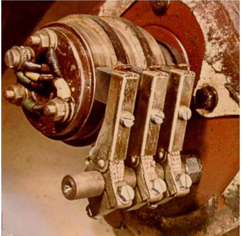
Fig. 26.3 Slip rings and brush holder of the motor shown in Fig. 26.2. The supply leads are protected according to IP65 and are still in working order.
