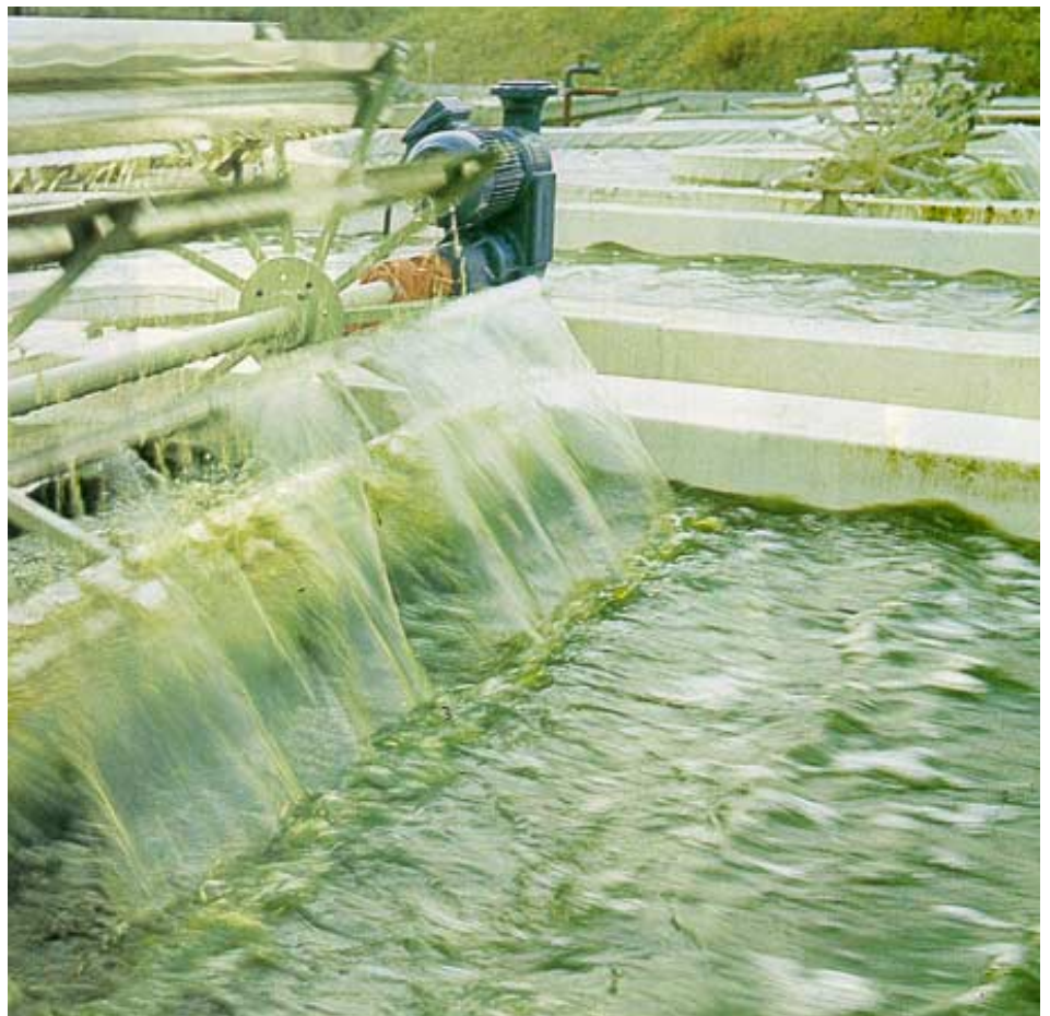
Fig. 26.29 Adjustable-speed geared motors driving aeration equipment at a settling tank.
