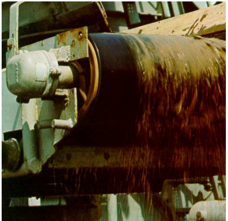
Fig. 26.14 Three-phase drum motor driving the conveyor belt of a river bed excavator.
