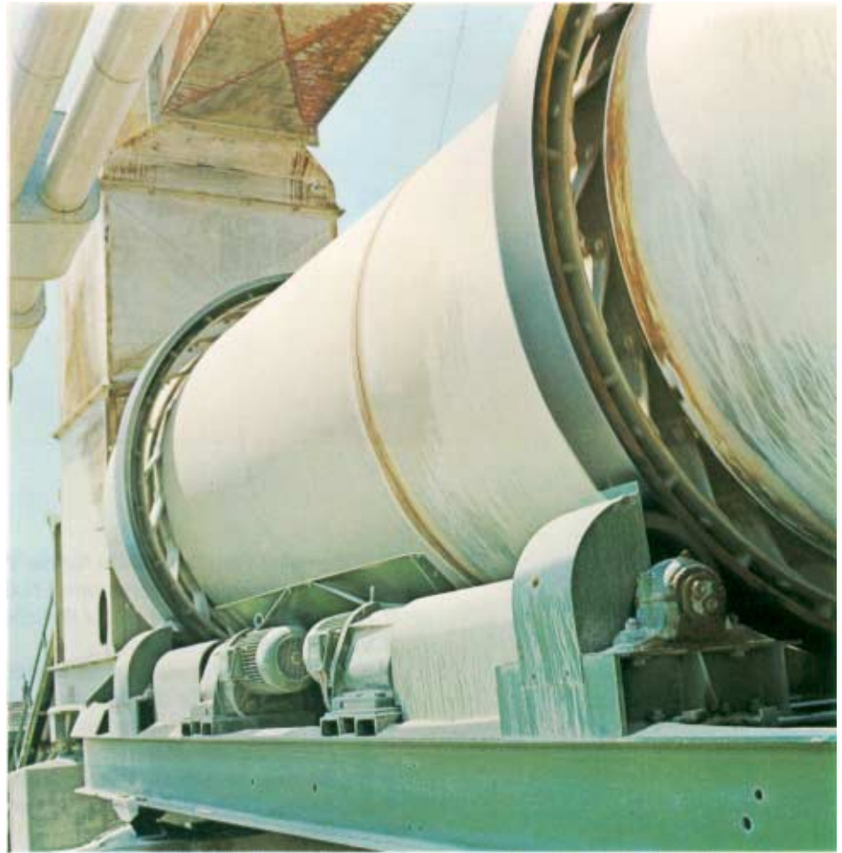
Fig. 1.1 Direct drive of a drying drum driven by three-phase geared motors
