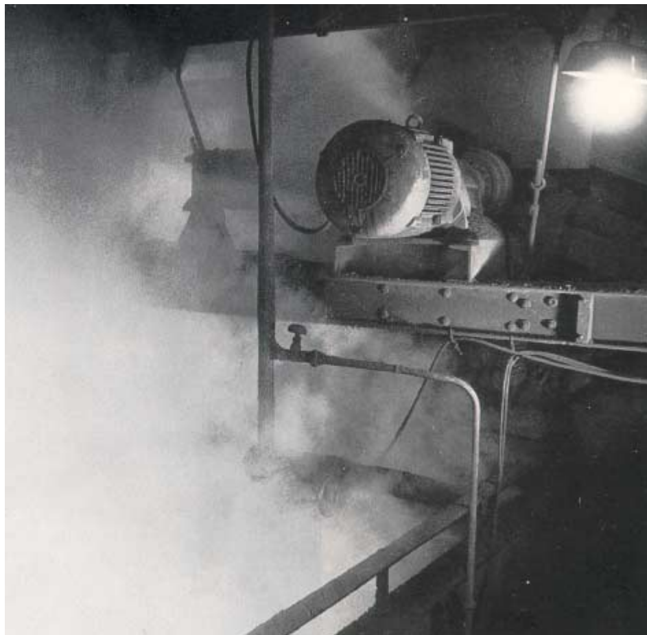
Fig. 26.16 Three-phase geared motor for driving a conveyor in a copper refining plant in a strongly corrosive atmosphere.
