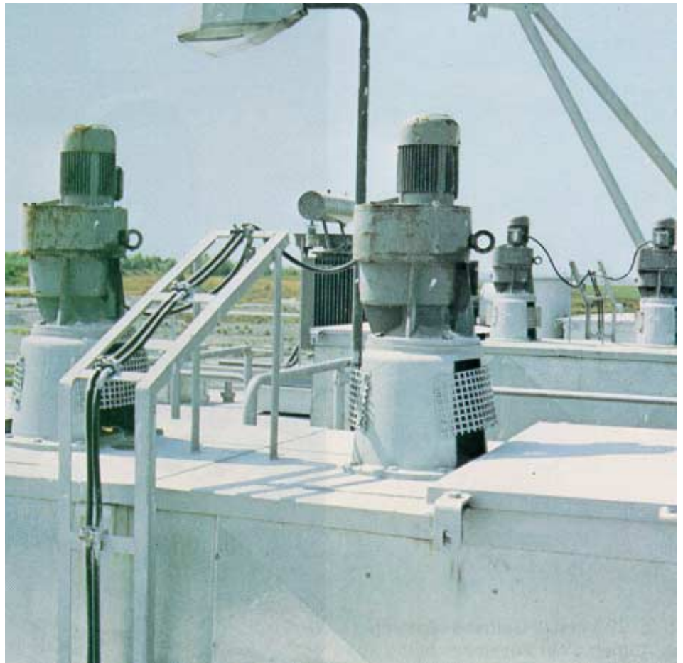
Fig. 26.25 Beaters for dust filters in a cement factory. Motors installed in open air.
